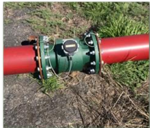
Flow meters record the amount of water diverted from a well or pump station
